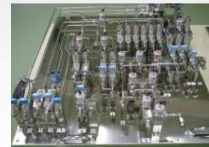
Gas supply panel
